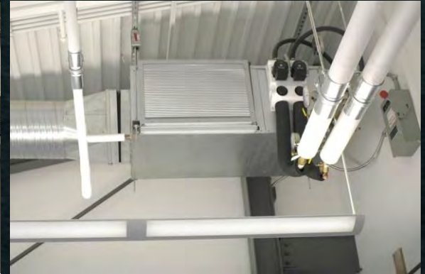
VSD Fans and VAV boxes
