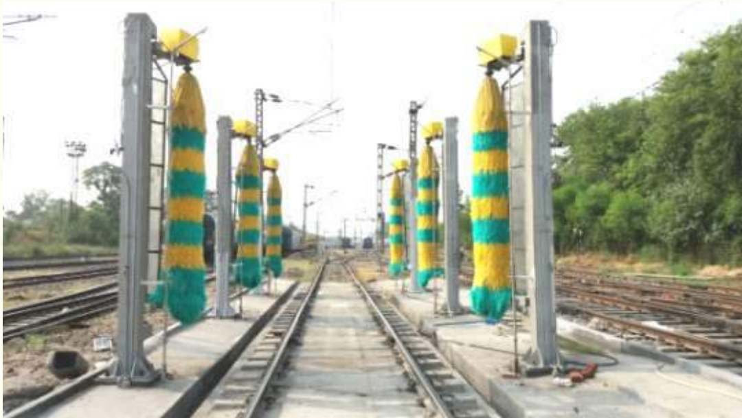
Automatic Coach Washing Plant with Water Recycling at Hazrat Nizamuddin Coaching Depot
