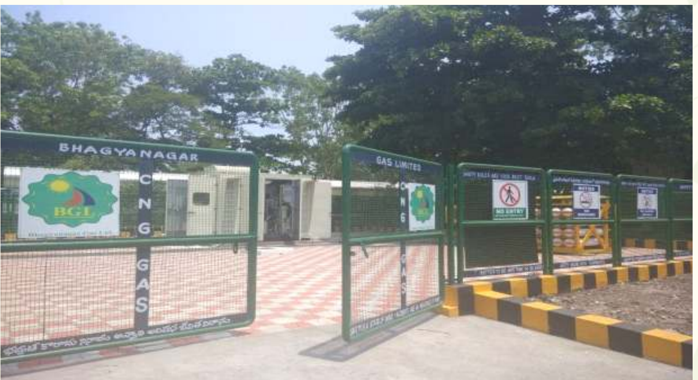
BGL Installation for CNG filling in Dual Fuel DPCs at DEMU Shed, Vijayawada
