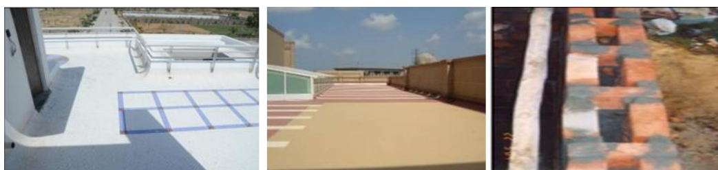
Figure 5: Use of High HRI coat on roof top and Use of Cavity wall on the western side of the buildings
