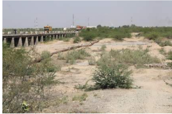
Bridge over Luni tributary. Note disused water pipeline north of NH-65 (March 2013)
