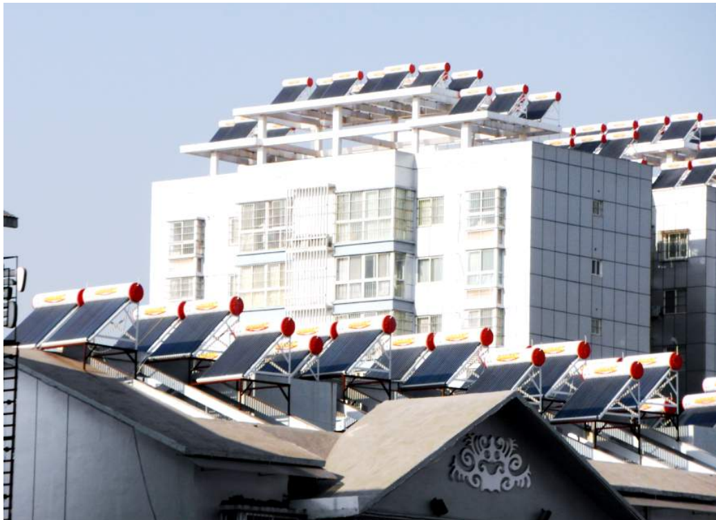
Figure 2- 8: Solar water heaters used in high density residential and commercial area
