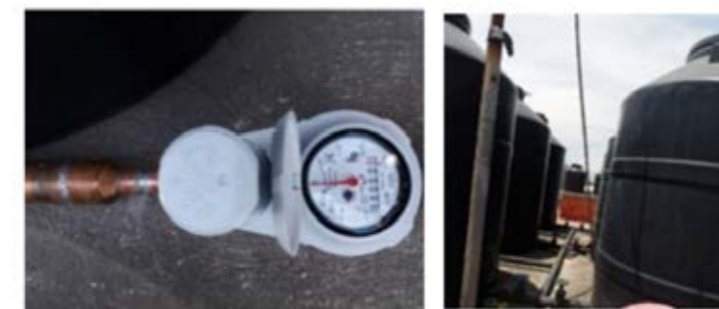
Figure 38. Micro meters installed at the low income housing of “Los Rojos” in Mexico City. Source: Josué Hidalgo, 2017
