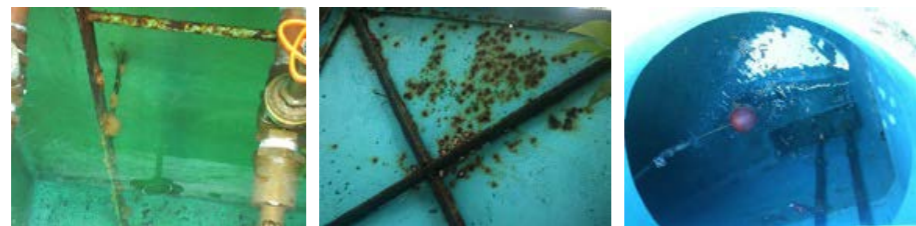
Figure 11. Inadequate conditions of some storage cisterns located at the University City. (PUMAGUA, 2012)
