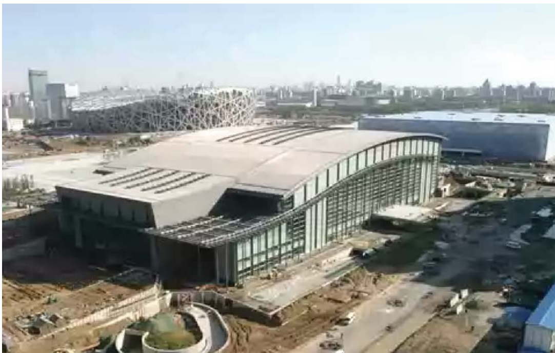
Illustration 49: Beijing Indoor Stadium during construction (front) with Beijing Olympic Stadium (behind) before the Olympic Games 2008 292
