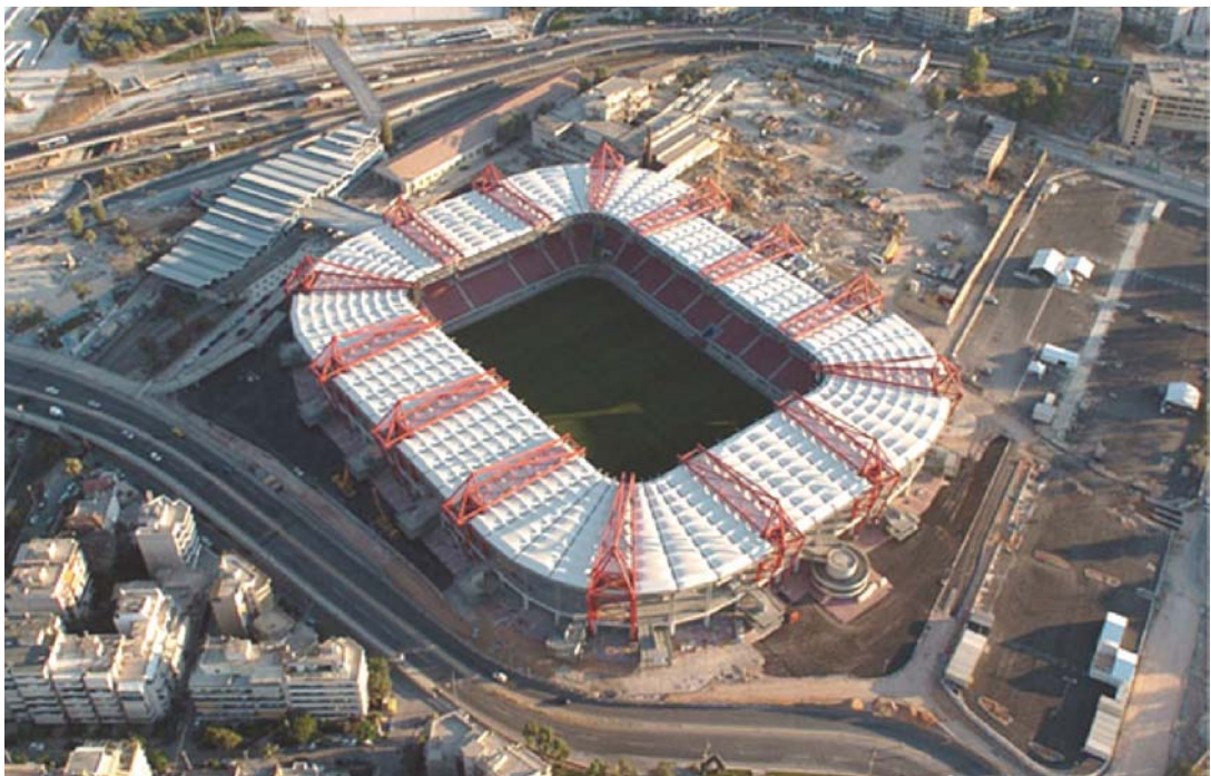
Illustration 41: Athens Football Stadium during construction on existing site before the Olympic Games in 2004. The original stadium was constructed 1895-1896 on this site for the world's 1 st Olympic Games 1896. xxxix Between 1952-1954 it was replaced with another stadium which was then demolished for this new stadium. 281
