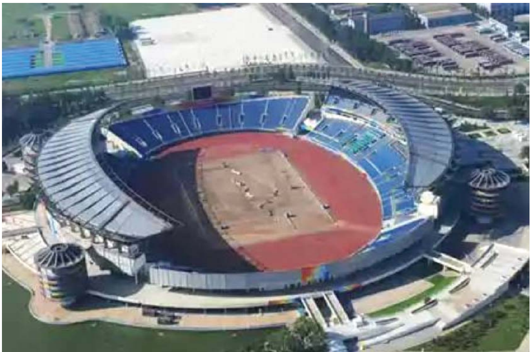
Illustration 52: Beijing Football Stadium with spectator capacity of 36,000 seats during construction of the new roof for the Olympic Games in 2008 296
