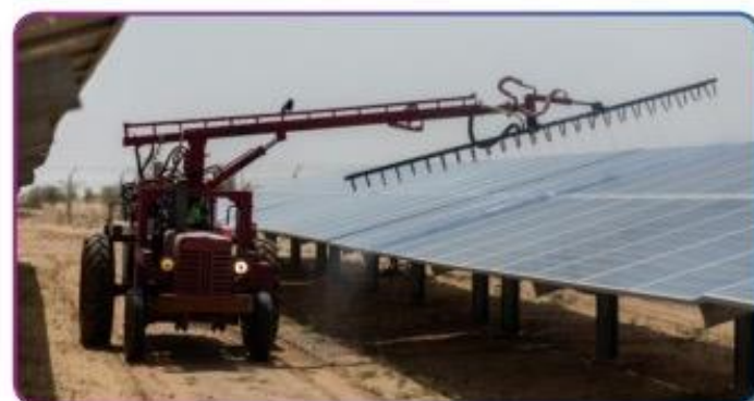
Innovation in Module Cleaning System (Semi - Automatic)
