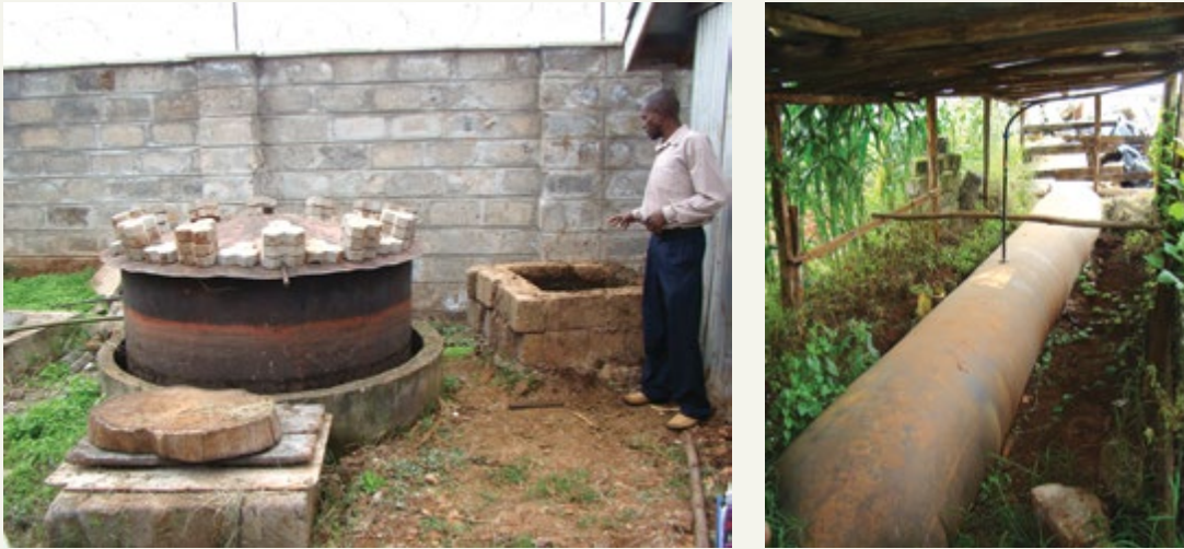
FIGURE 2.19. Small on-farm anaerobic digester in Kenya using manure from a 4 cow dairy herd with butanol gas storage bag.
