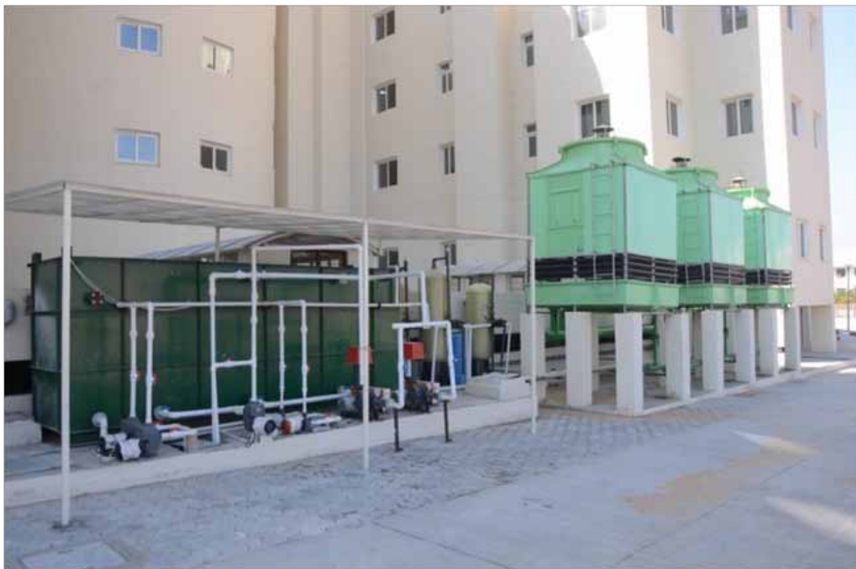
Figure 16.7: Cooling towers for the centralized high-efficiency water-cooled chiller system (right) with the waste water treatment system (left)
