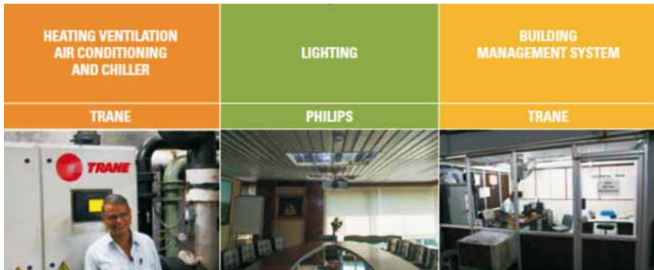
Figure 2: Energy-efficiency Technologies Installed
