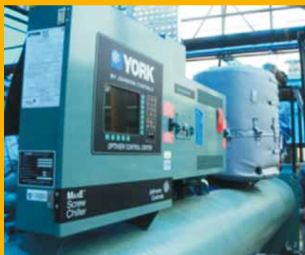
Figure 1: Replacement of Air Cooled Chiller to Recycled Water Cooled Chiller at the ITC Plant in Bangalore
