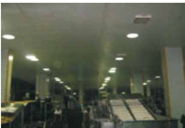
Figure 1: Sky pipe lighting at the Food Processing industry
