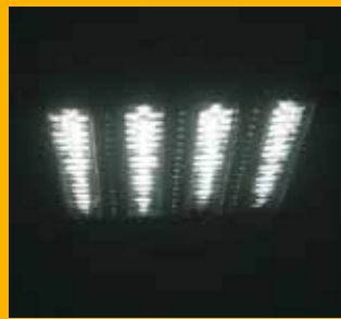
After with 4X14Watts T5 light fixture
