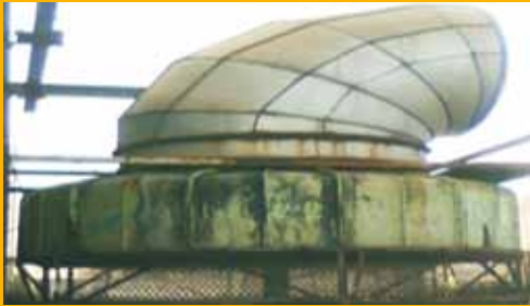
Forced Draft Cooling Tower
