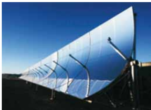
Parabolic Trough Collector (PTC)
