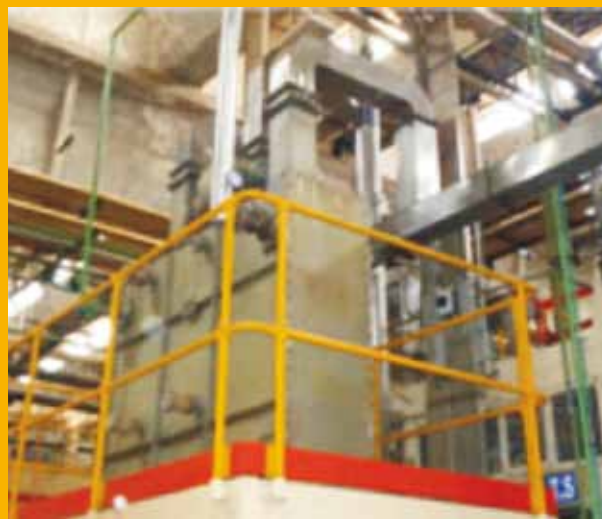
Figure 2: Heat Recovery from Process Exhaust at the Process Department in ITC Bangalore
