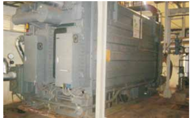
Figure 1: Vapor Absorption Machine based chillers at Food Park, Jain Valley, Shirsolli Road, Jalgaon
