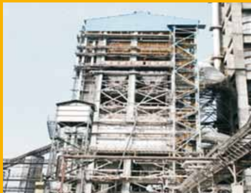
Figure 1: Installation of Waste Heat Recovery system to trap the waste heat from preheaters and Air Quenched Coolers (AQC) of Clinker manufacturing pyro process to trap the waste heat
