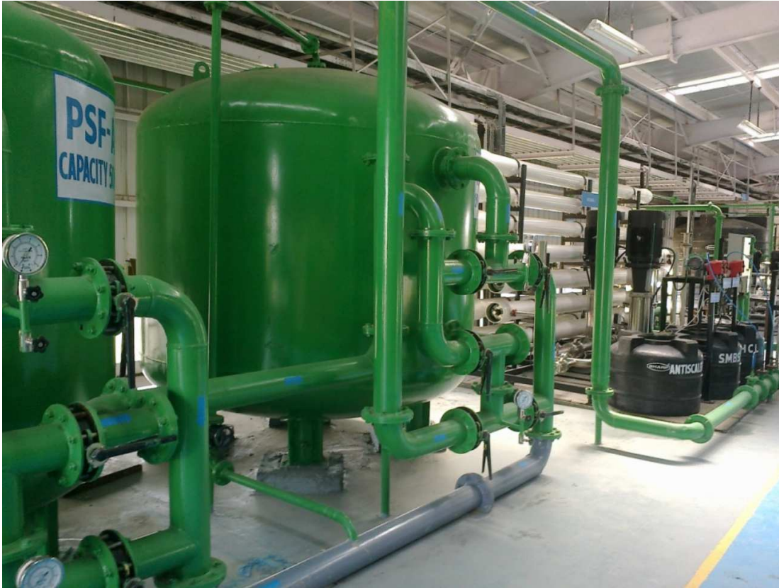
Tata Motors, Pantnagar - Capacity - ZLD-100m 3 /hr-Filtration, 3 Stages RO
