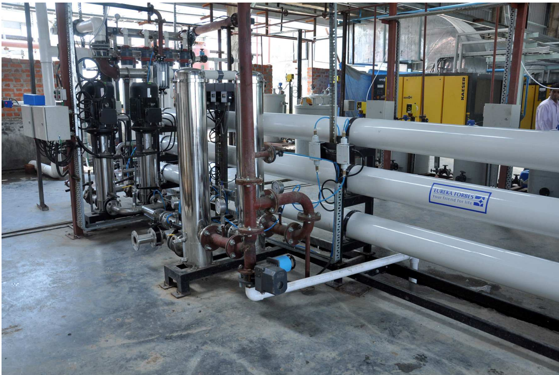
CEAT Limited - Capacity - ZLD-UF & RO - 40m 3 /hr
