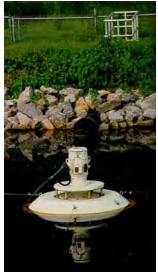
Post-aeration is essential for compliance with the effluent standard for dissolved oxygen.
