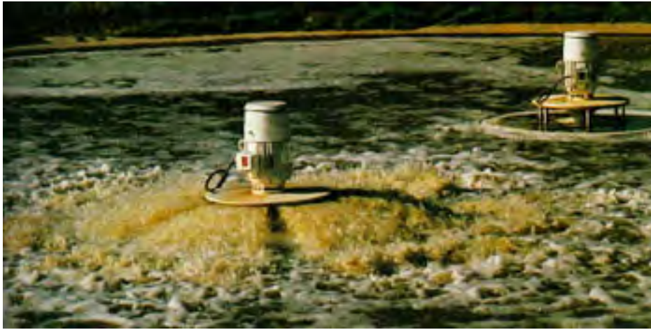
Post-aeration is essential for consistent compliance with the dissolved oxygen permit limit of 6.0 mg/l.
