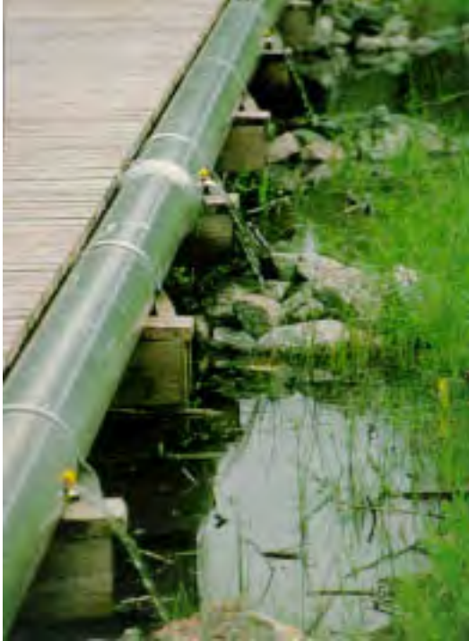
Aluminum pipes distribute the treated effluent.
