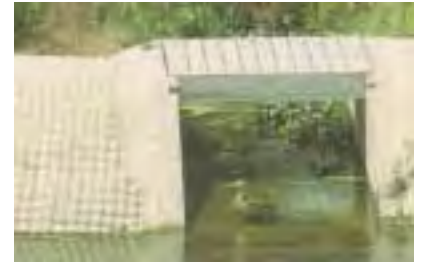
Weirs located along berms covered with grout-filled fabric revetments distribute flow into the cells 2 and 3.
