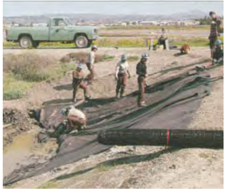
Biodegradable mesh was laid on banks near inlet and outlet structures during construction.
