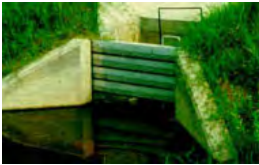
Outlet weir structures allow water level control for adjustment of hydraulic retention time.
