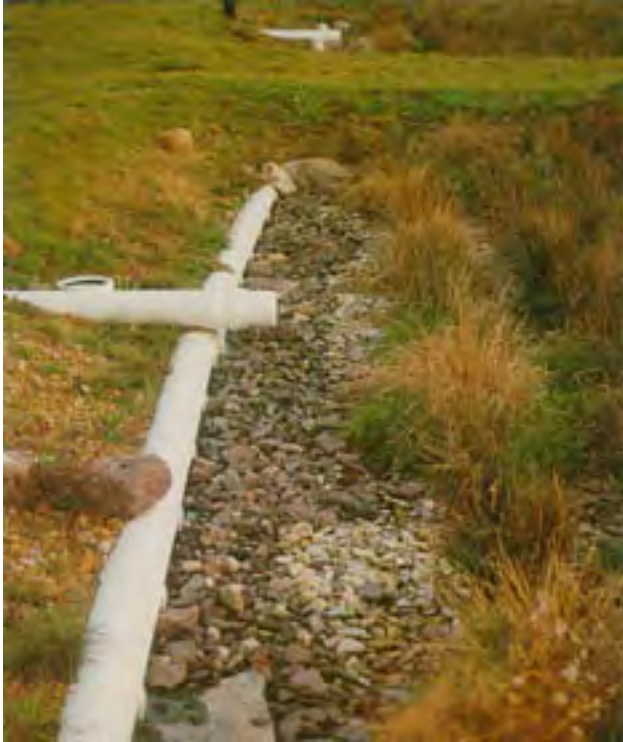
A recently expanded Subsurface Flow constructed wetland system serves the small community of Monterey in Highland Co., Virginia.
