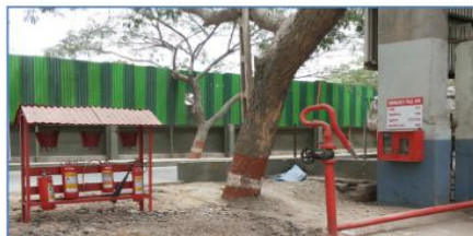
Proper Fire Hydrant System
