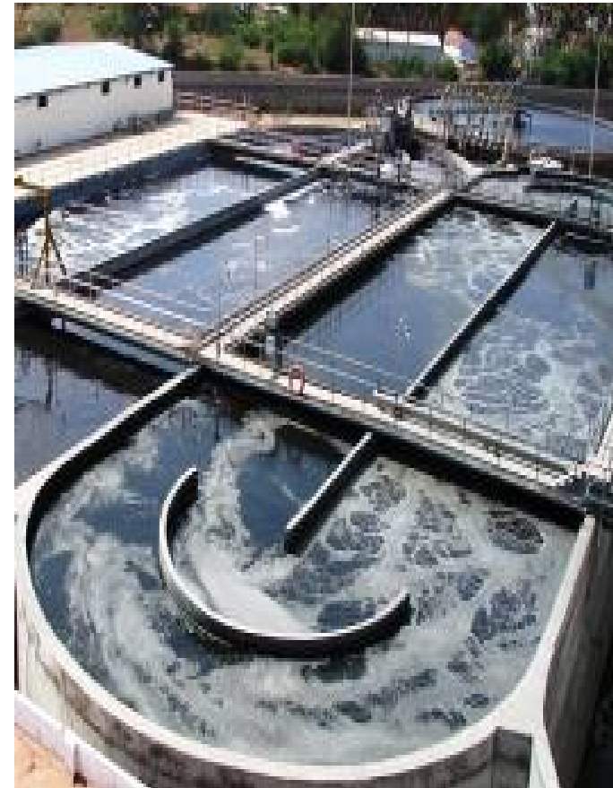
Fig: Biological Oxidation Tank equipped with diffused aeration system at Tirupur site
