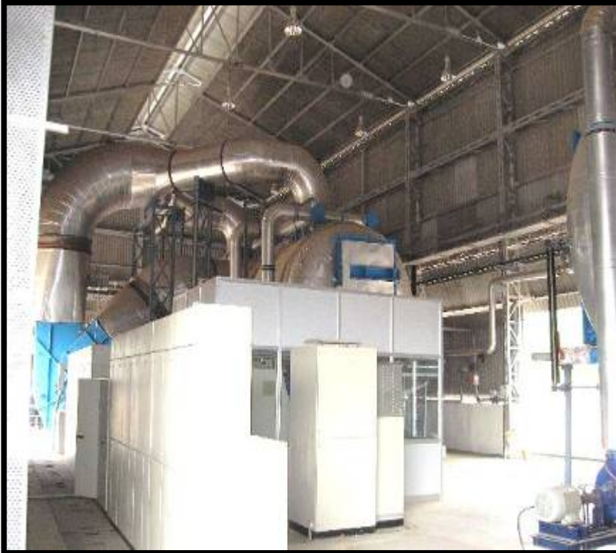
Fig: MVR type Evaporator System installed in all CETPs
