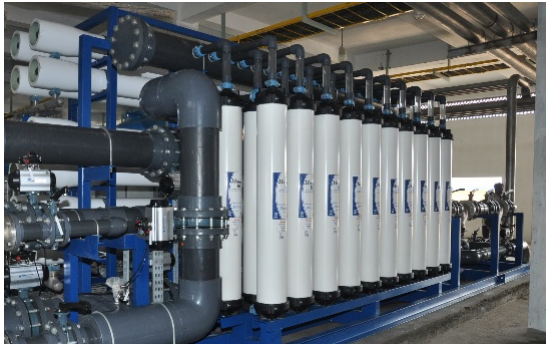
Figure 7. Ultrafiltration at RANITEC
