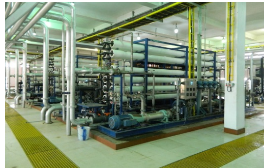
Figure 8. Reverse osmosis at RANITEC
