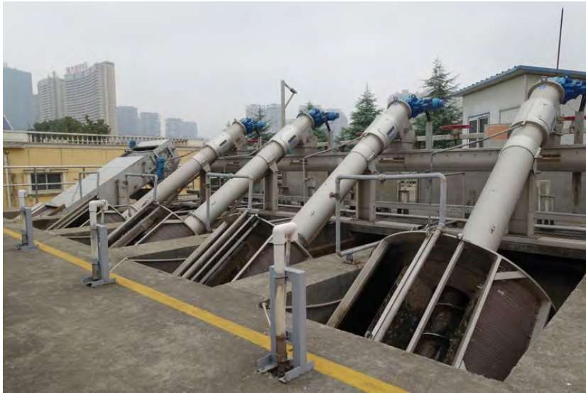
Figure 13: Fine screens in a sewage treatment plant
