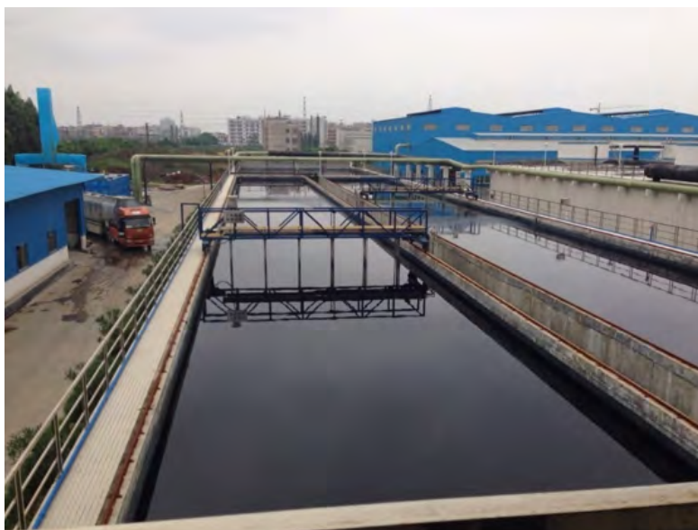
Figure 19: Rectangular sedimentation tank in a textile effluent treatment plant, China
