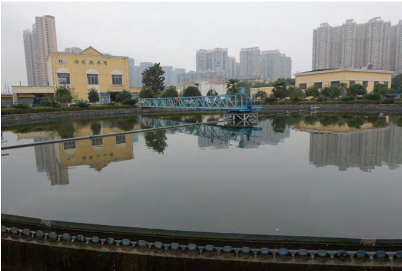
Figure 47: A photo of a circular clarifier
