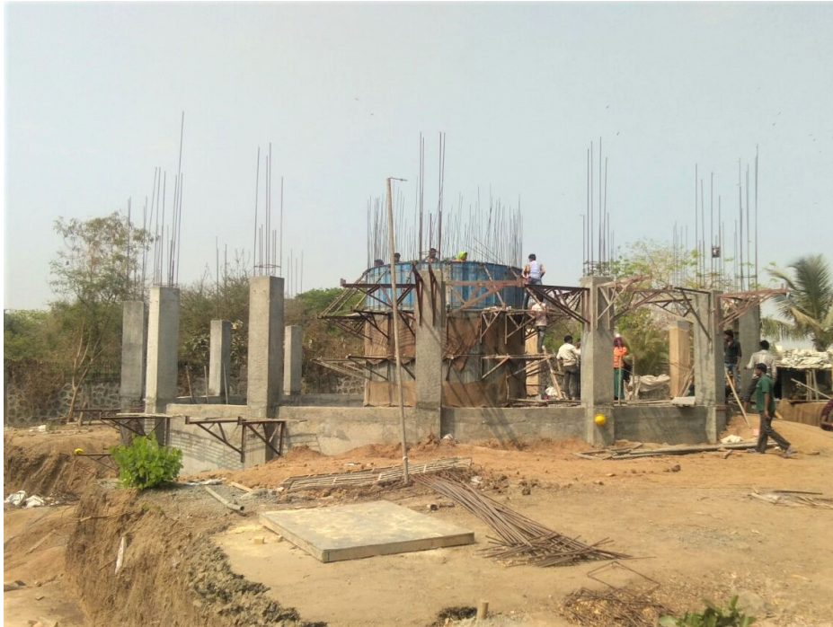
Dirty Water Sump (WTP)
