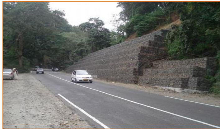
Figure Error! No text of specified style in document..5: Gabion Walls for Slope Protection
