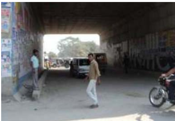
Figure 21: Underpass at Km 78.350 Footpath should be provided on service road at underpass location.
