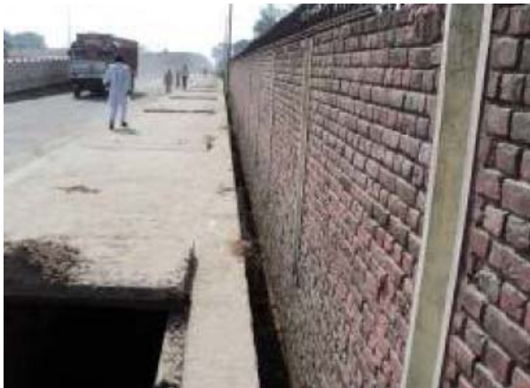
Figure19: Underpass at Km 78.350 • Drain should be covered.
