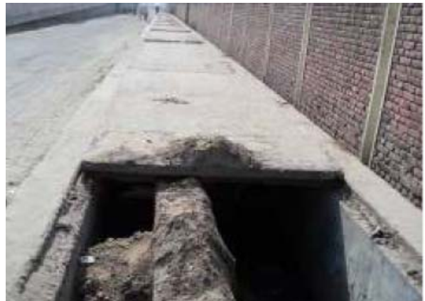
Figure 20: Underpass at Km 78.350 • Gap between wall and drain should be filled.
