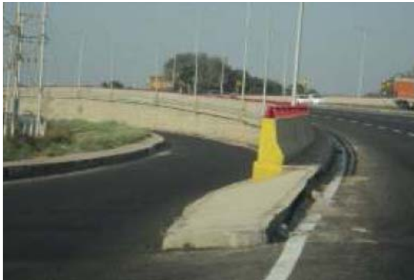
Figure 25: Service Road & Start of Underpass at Km 121.800: Hazard Marking and Chevron Marking are missing.
