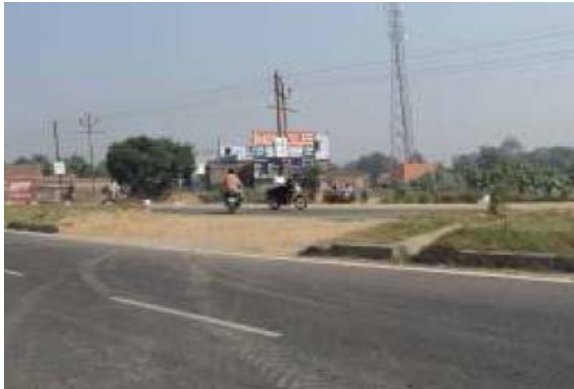
Figure 15: Unauthorized Median Opening at Km 75.160
