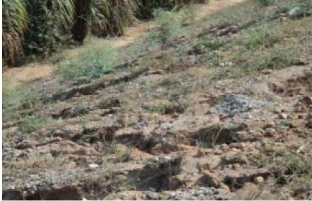
Figure 23:Embankment of ROB Approach at Km 87.600: Rain cuts were seen on slopes as the slopes were not protected.
