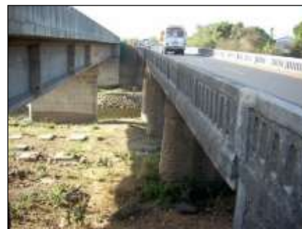
New and Old Bridges over Wanki on NH-48 showing difference of level
