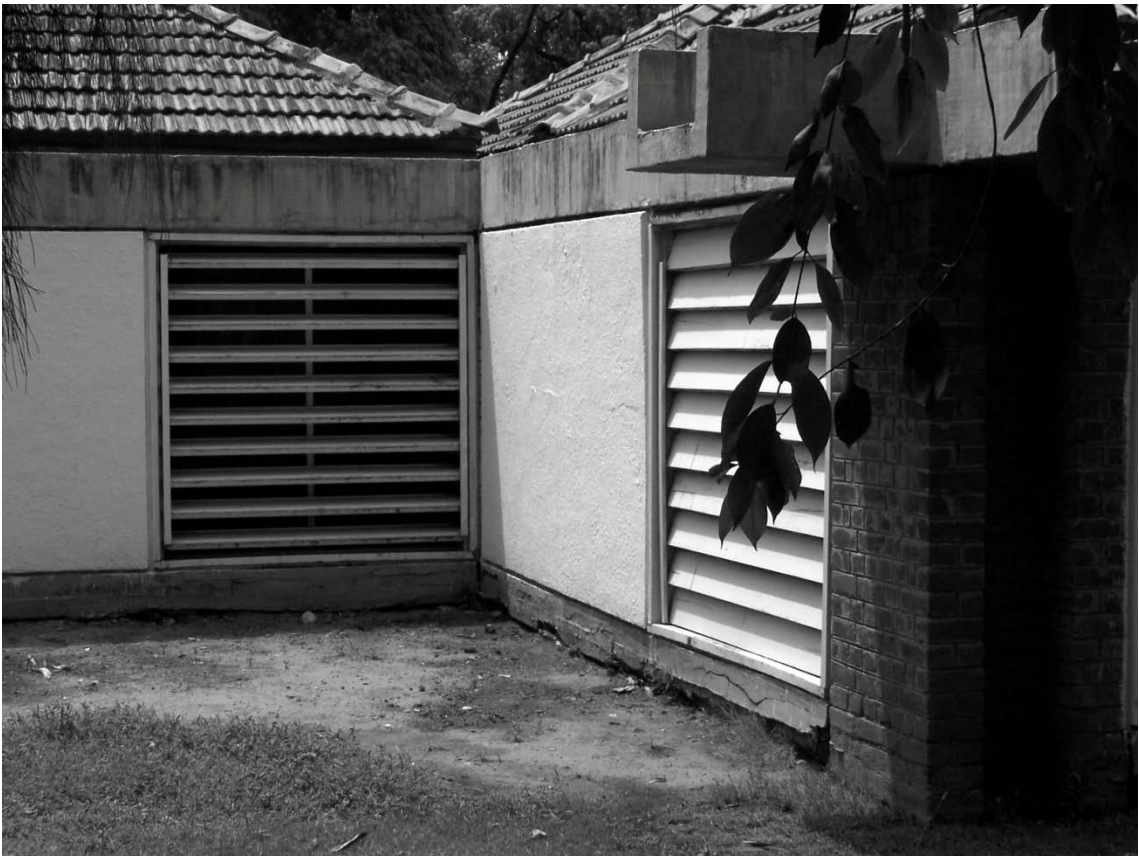
Figure 2.23: Operable louvers allowing control over sunlight penetration and airflow: Gandhi Smarak Sangrahalaya, Ahmadabad; Charles Correa
