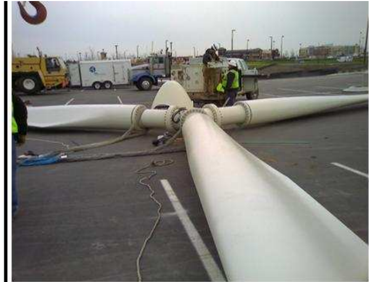
Crews assemble the wind turbine rotor and prepare to hoist it to the top of the turbine.
