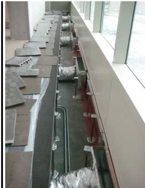
The under-floor displacement ventilation system can be seen here under raised floor panels.
