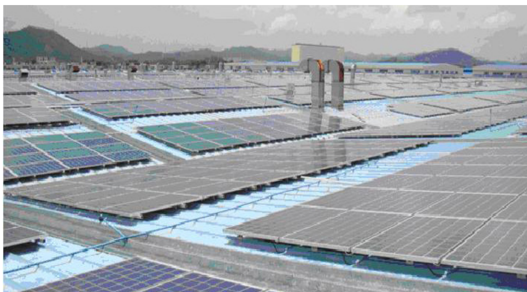
Rooftop Solar Distributed Photovoltaic Power Projects
