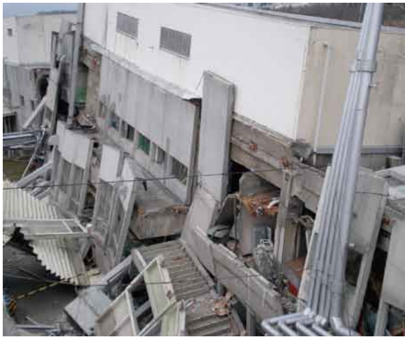
Factory partially destroyed by the quake in Sukagawa City, Fukushima Prefecture
