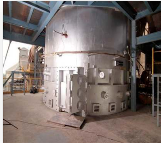
Fig: Hot disc reactor at Vasavadatta Cement.
