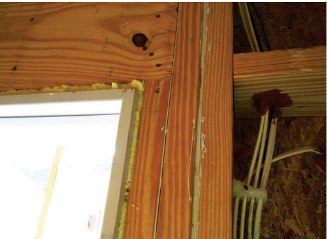
▲ Figure 15.2 High standards for air sealing were implemented on this project. (Courtesy of Lend Lease)
