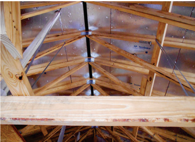
▲ Figure 15.3 Radiant barrier roof sheathing was used to reduce the radiant heat absorbed into the home. In colder climates, it is often more cost-effective to add more insulation instead of a radiant barrier. (Courtesy of Lend Lease)
