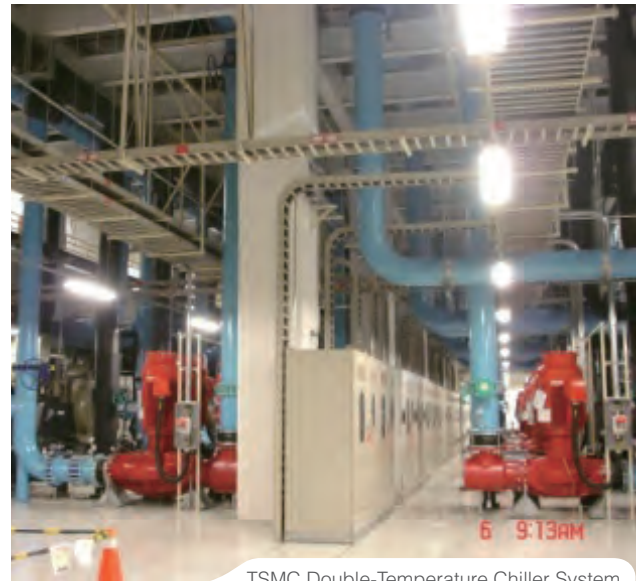
TSMC Double-Temperature Chiller System
