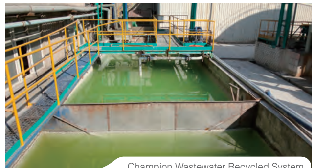
Champion Wastewater Recycled System
