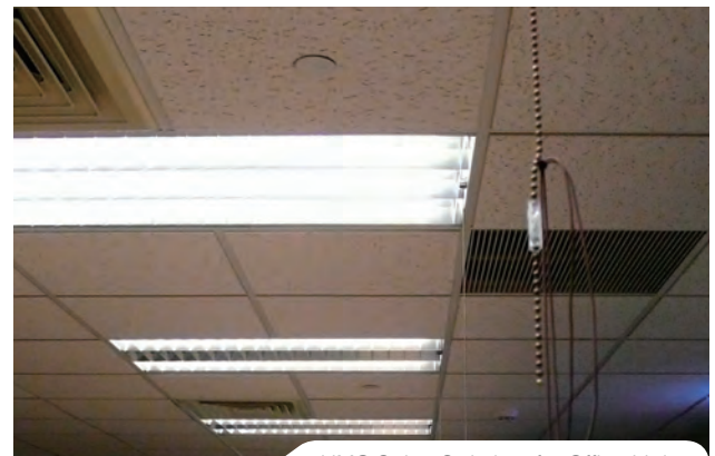
UMC String Switches for Office Lights
