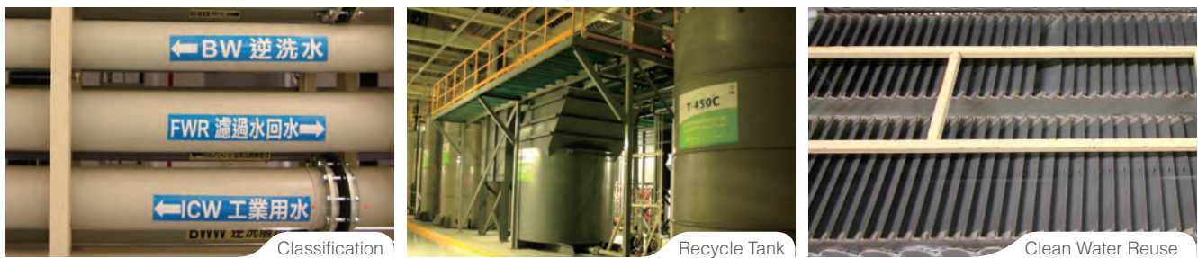
TSMC Wastewater Collection & Treatment Systems (Source: TSMC Corporate Social Responsibility Report, 2012)
