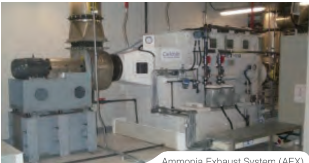
Ammonia Exhaust System (AEX)
