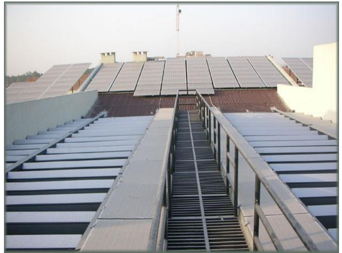
Figure 2: Solar Power generation at Akshaya Urja Bhawan
