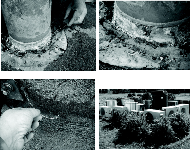
Figure 1 Roof case study: aluminum drains are perforated at the base (top pictures); lack of anti-root membrane leading to root growth and deterioration of the waterproofing membrane (bottom left picture); and mechanical equipment located in a cluster (bottom right picture).
