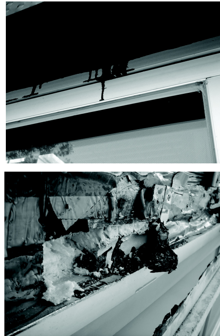
Figure 2 High performance window case study: Bitumen streaks on the window frame (top); disintegrated flashing membrane but fairly intact sealant with water accumulation and infiltration at head of the window (bottom).
