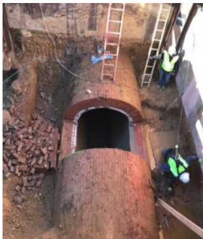
The removal of the top of the sewer outside the building for the sewer heat exchange. Photo Courtesy of Skanska.
