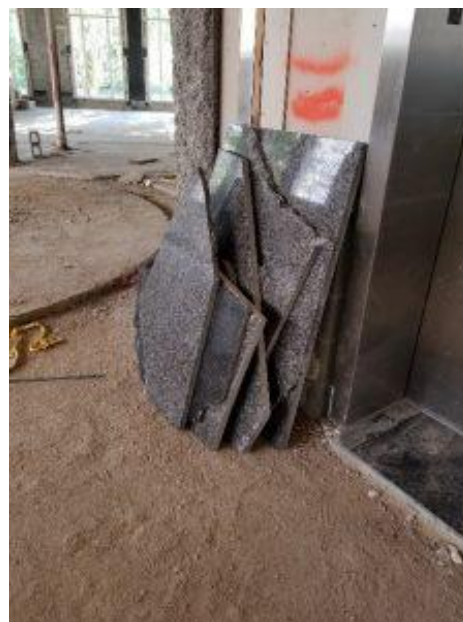
Stone from the first floor lobby that was saved for reuse in the terrazzo material. Photo Courtesy of AGU.
