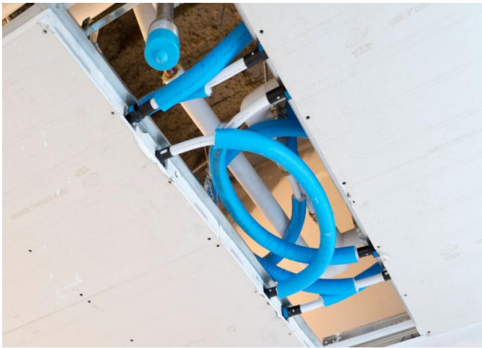
Direct current electrified grid in the ceiling. Photo Courtesy of USGBC.
