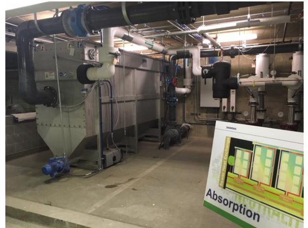
Settling tank for the municipal sewer heat exchange. Photo Courtesy of AGU.
