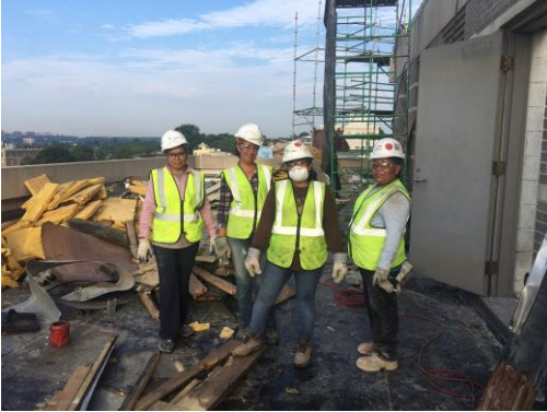
Female members of the demolition crew on the roof. Photo Courtesy of AGU.
